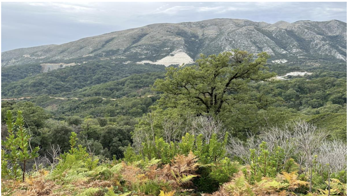
Figure 5: The construction of the pipeline route in the middle of the oak forest © U. Eichelmann
